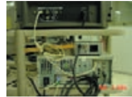
Step 3: Recording Device to Monitor Connection
